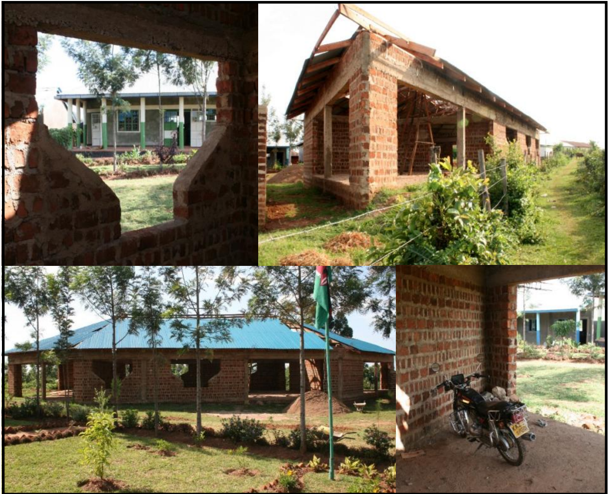
Mwituha Library under construction February 2010. See our video tour of the campus and library at www.kijana.org/video
