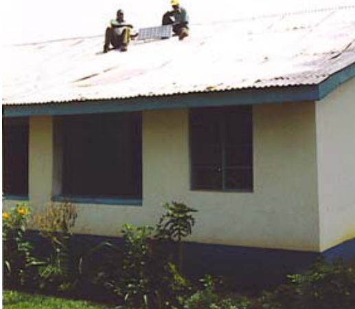
Ben Asembo and assistant of Village Electrical, installing solar panel atop Essaba Secondary building, allowing school to harness free energy.
